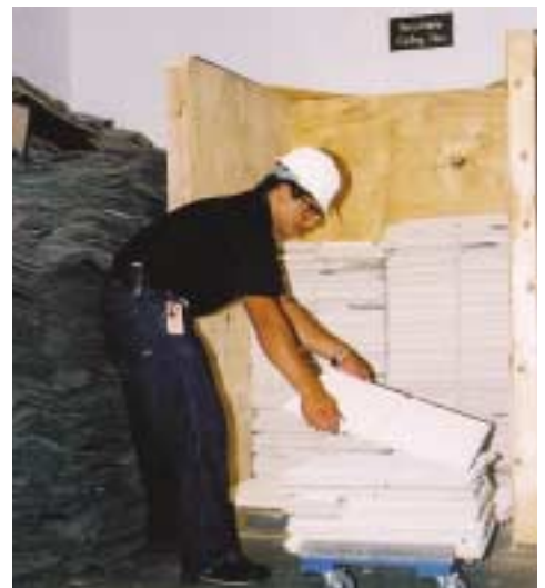
Following removal, old ceiling tiles are stacked and stored at the World Bank facility prior to pick-up by Capitol Building Supply, the ceiling distributor. Recyclable carpet tiles are seen on the left.
